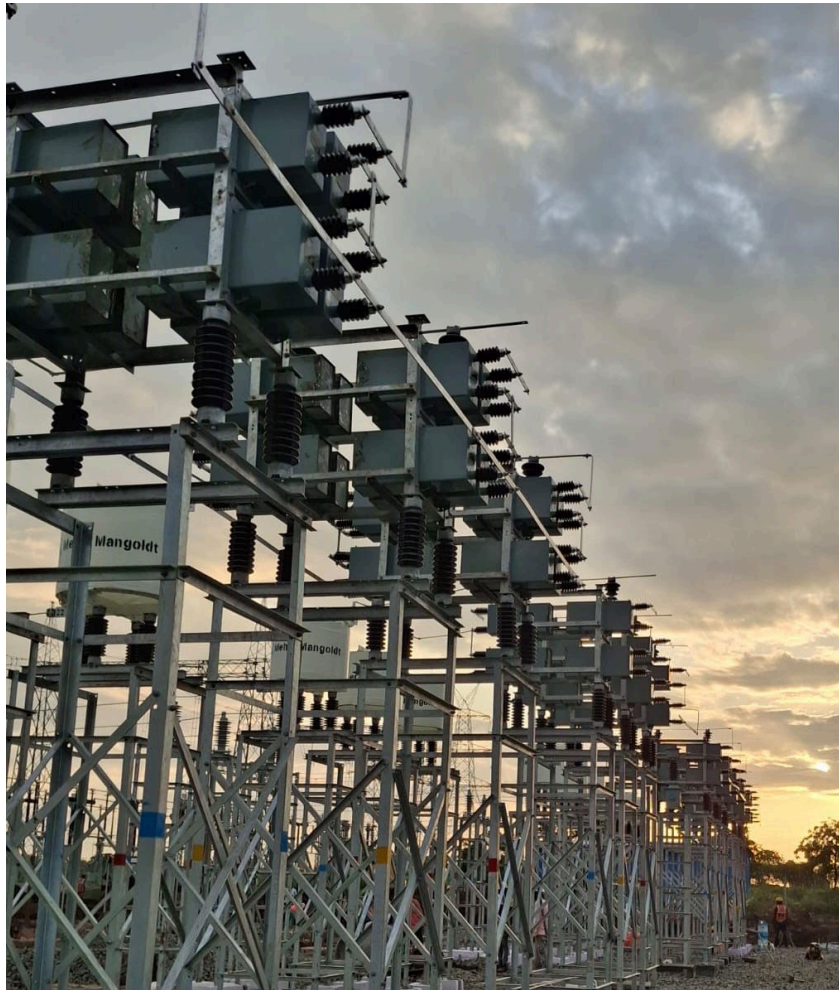
CosPower's Capacitor Banks at a Steel Plant
