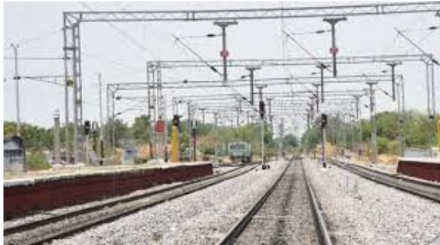
Railway Traction Substation
