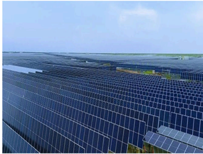
300 MW Solar Power Plant
