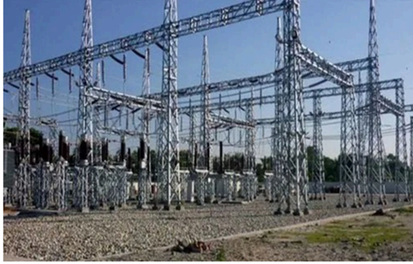
Power Utility's 132 kV Electrical Substation
