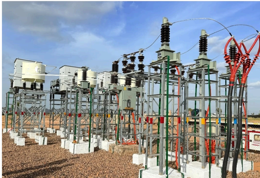
Harmonic Filter in a Solar Generation Plant
