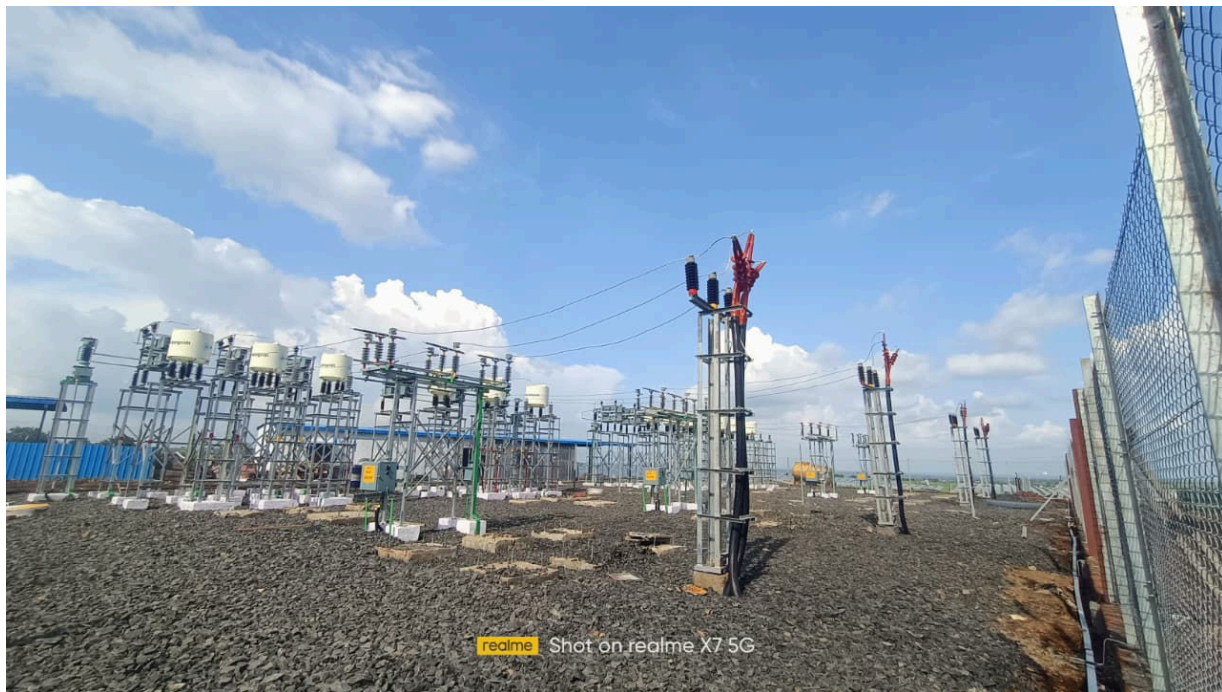
CosPower's Capacitor Banks Solar Plant
