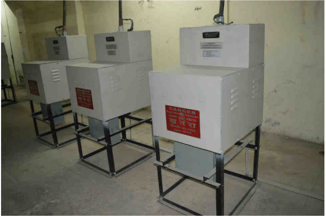
HT CAPACITORS CONNECTED ACROSS LARGE MOTORS
