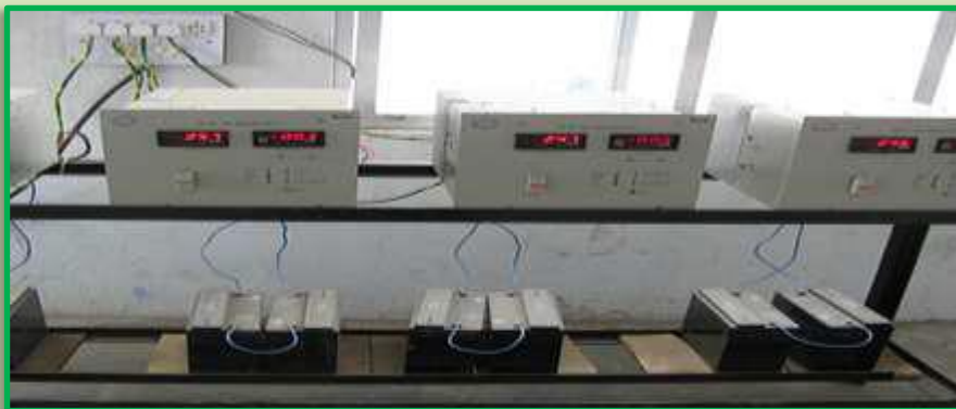
Battery and Battery Chargers
