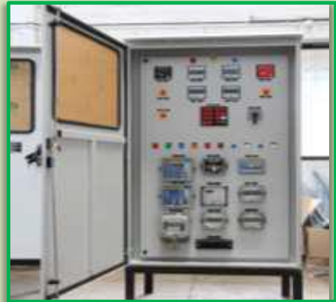
Control and Relay Panels
